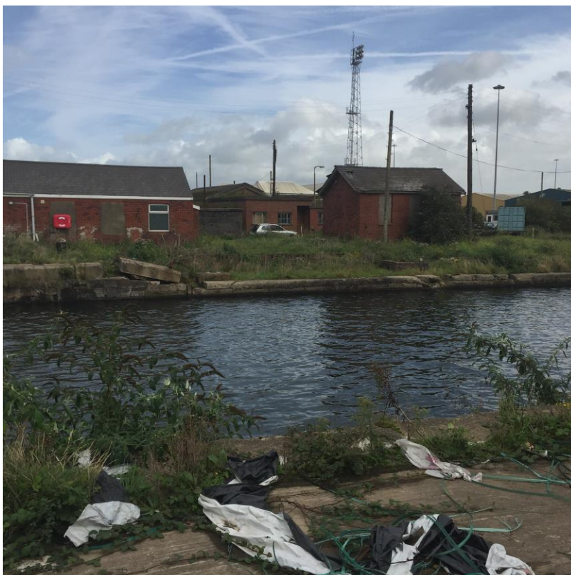
Figure 3-2 Missing Coping Stones - Junction Cut
