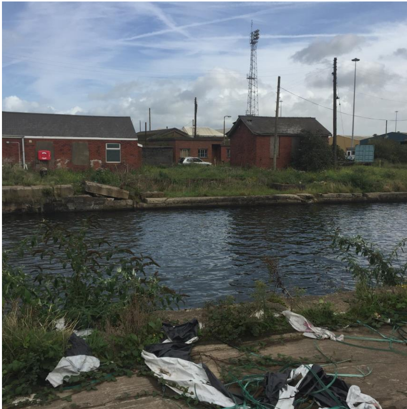
Figure 3-2 Missing Coping Stones - Junction Cut
